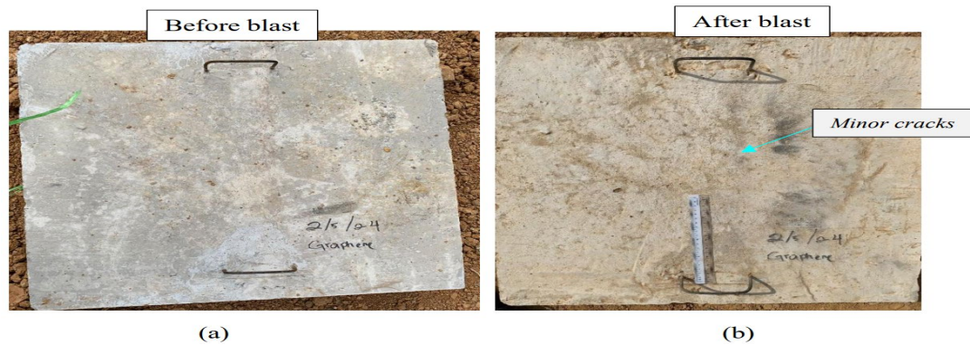
Figure 5 (a) & (b). Photographs of cracked NRC and GRC slabs.
